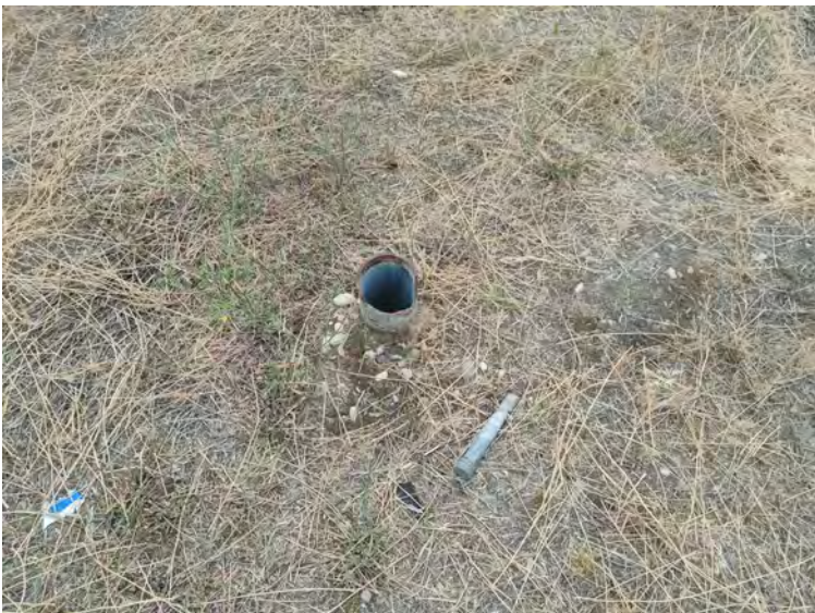
PHOTOGRAPH #9: THIS PHOTO SHOWS THE UNCAPPED WELL.
